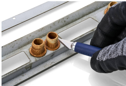
Continue with the rubber sleeves. Remove these with the scalpel as well.
